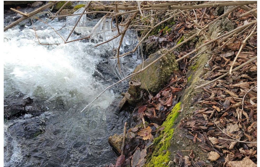
Cold Water Discharge Valve
