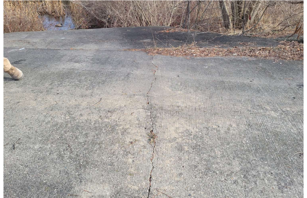
Concrete Cracking in Auxiliary Spillway
