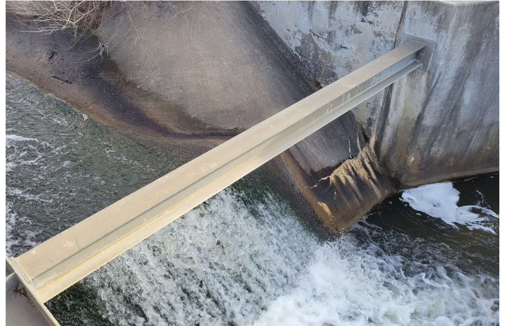
Concrete Cracking and Efflorescence Along East Wall
