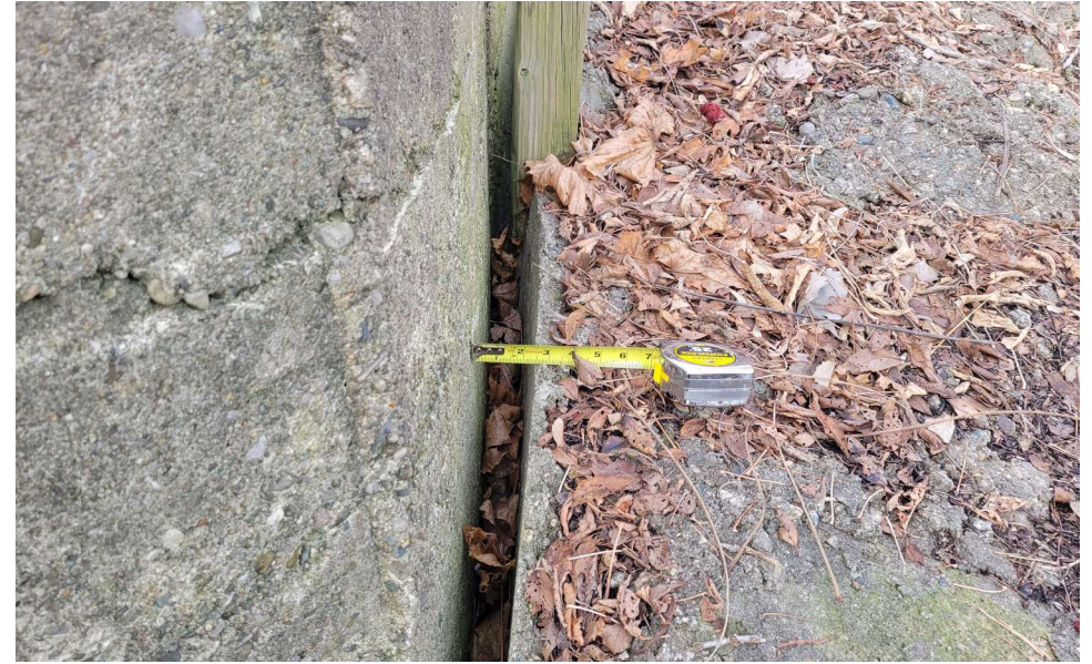
Approx. 2.5" Gap between Downstream Headwall and Wingwall on Auxiliary Spillway
