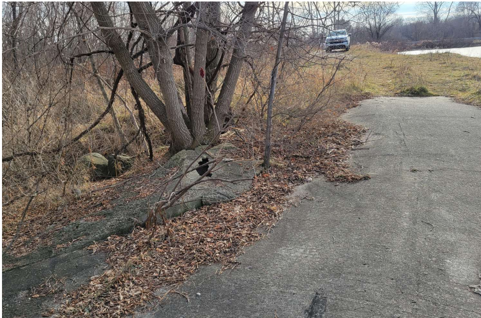
Tree Growing Next to Auxiliary Spillway
