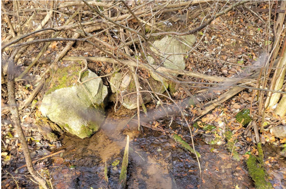
Seepage through Embankment
