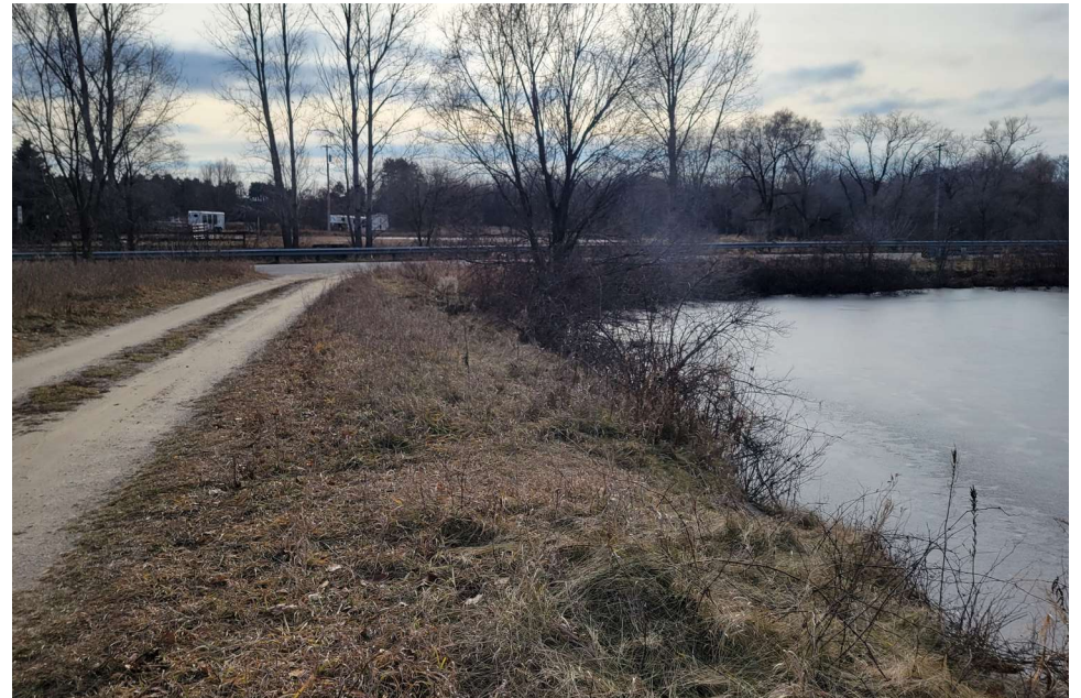
Looking South at Brush and Tree Growth Along Embankment
