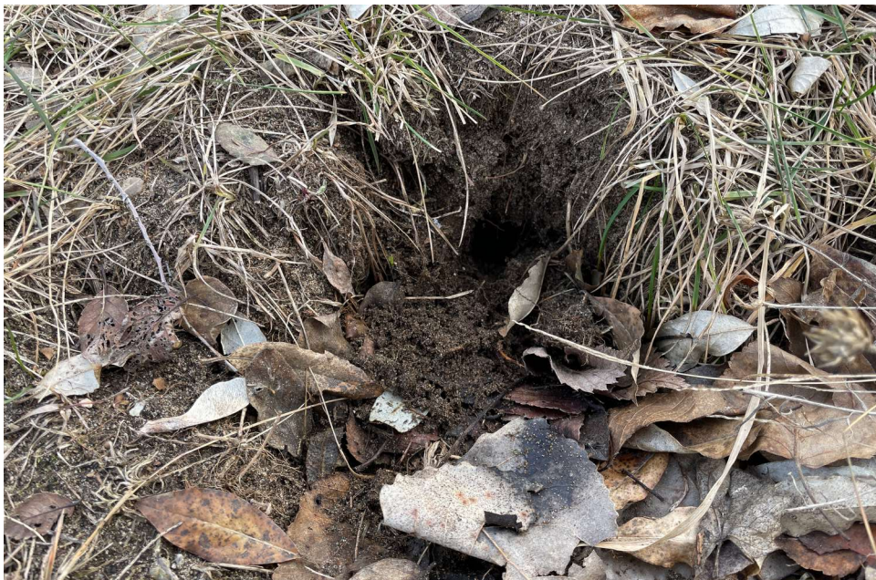
Rodent Hole in Embankment
