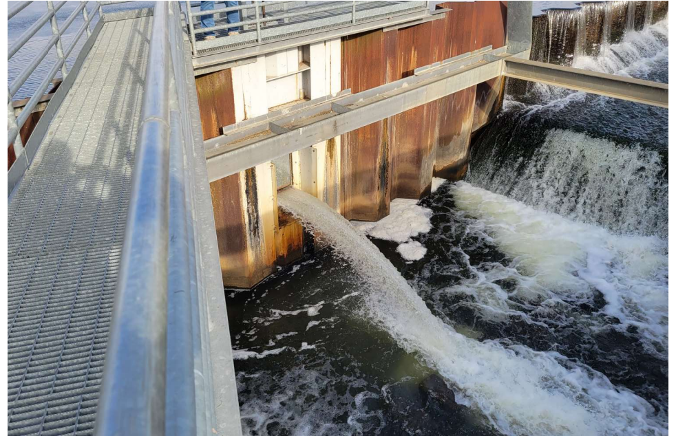
Sluice Gate Operational
