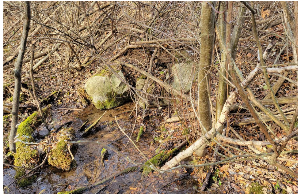
Seepage through Embankment at Eastern End of Embankment
