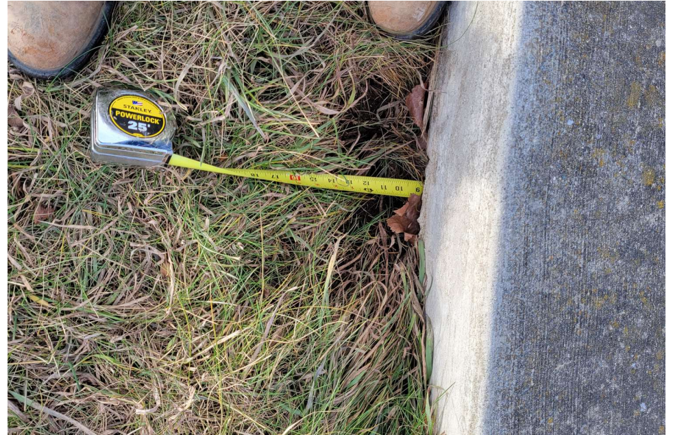
Void Underneath Slab on Eastern End of Structure
