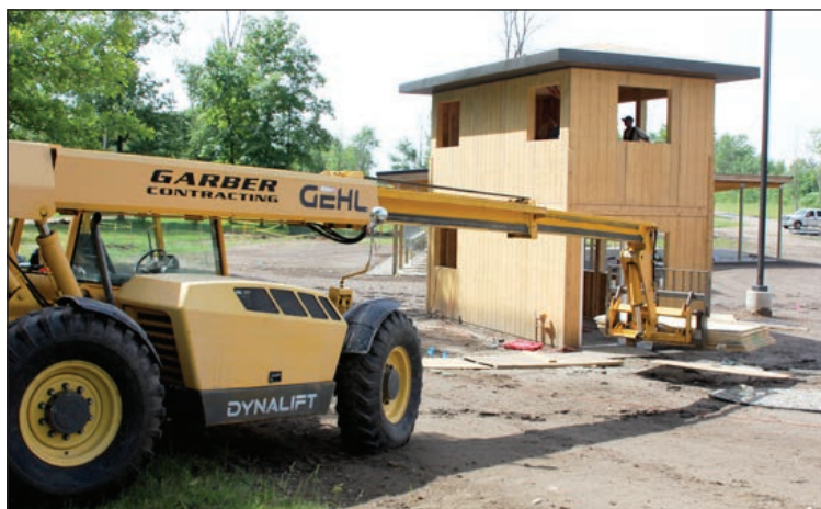
Garber Contracting works on the electrical, and the newly-constructed emcee/powwow committee stand in time for the 30th annual Saginaw Chippewa Powwow.
